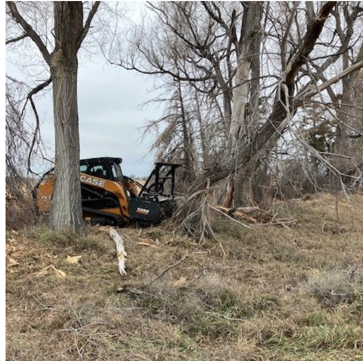
The Resource Conservation Department has been working on implementing a new Windbreak Renovation Strategy. They are using a Forestry Drum Mulcher and a tracked compact loader to create planting paths through existing degraded or non-functional windbreaks.
